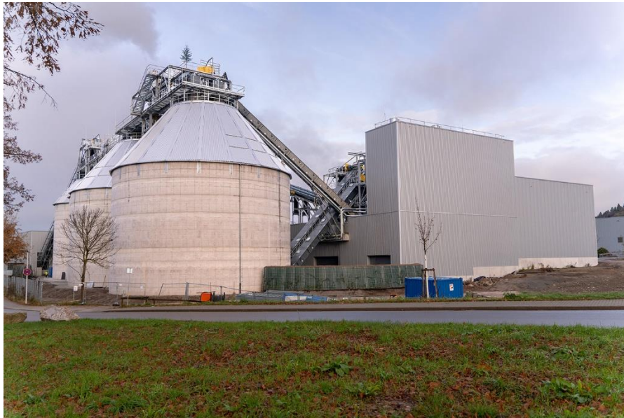
Figure: Right in the home stretch – the conversion work on the Koehler Group combined heat and power plant in Oberkirch.
